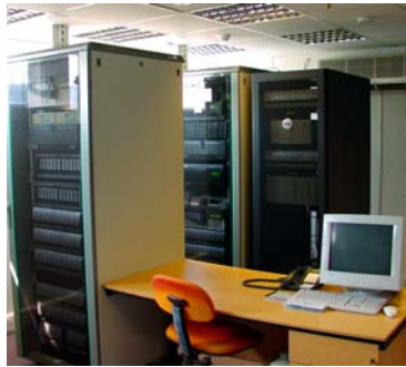
Storwave's Hosting Facilities are located in Bristol and Aldershot, UK
